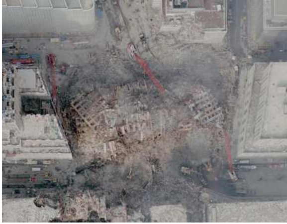
Figure 1.7 WTC 7 debris pile (NOAA, September 23, 2001).
